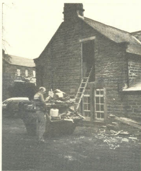
Work in progress on creating a new room for the Dore Village Society above the kitchen at the Old School.
