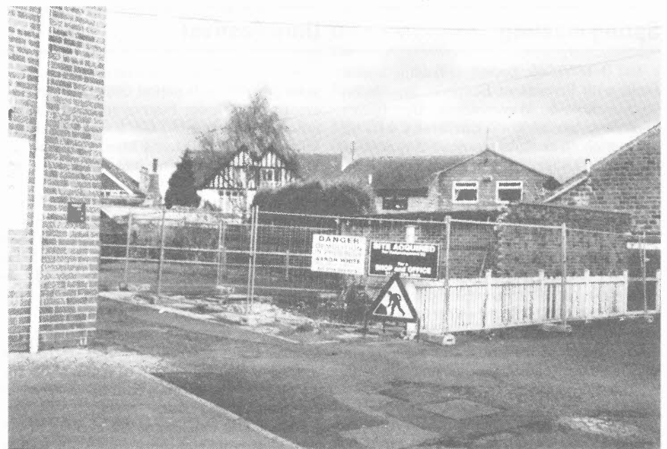
Site of the Dore public toilet block, after its clearance ready for the building of new offices.
