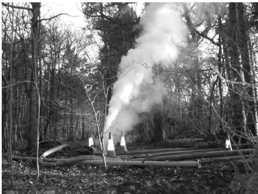
Dore Geothermal project? Steam venting from a manhole in Ecclesall Woods during the re-lining of sewers. Picture provided by Richard Farnsworth..
