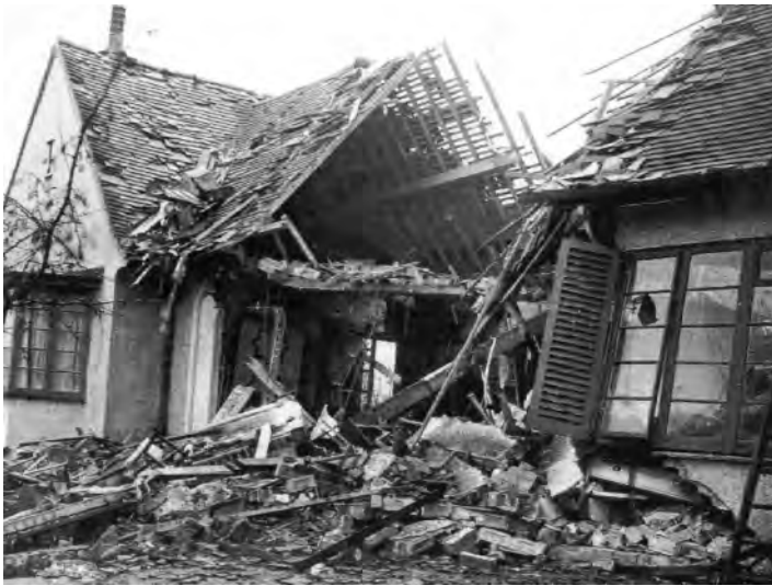
Ianford, Church Lane, the bungalow belonging to Mr Hartley after it was bombed in January 1941.
