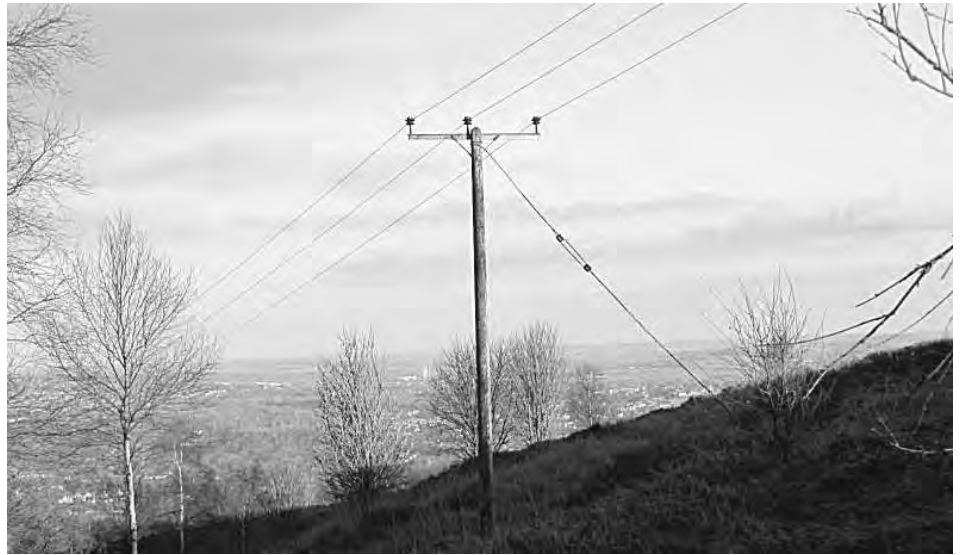
The high voltage power line that strides inflexibly across Blacka Moor.
