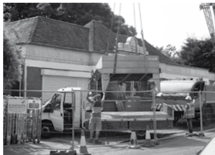
New refrigeration plant being lifted onto the Co-Op roof as part of the refurbishment work
